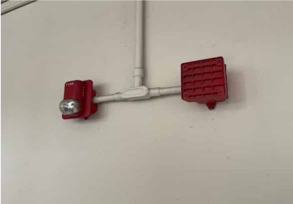
Bldg D Fire Alarm System Equipment
