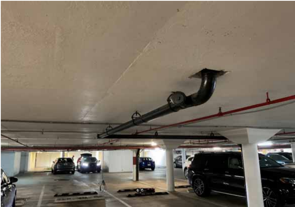
Garage Plumbing lines
