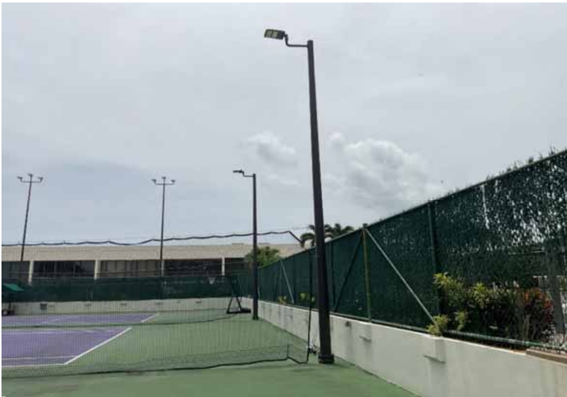
Tennis Court Light Pole & Fixture
