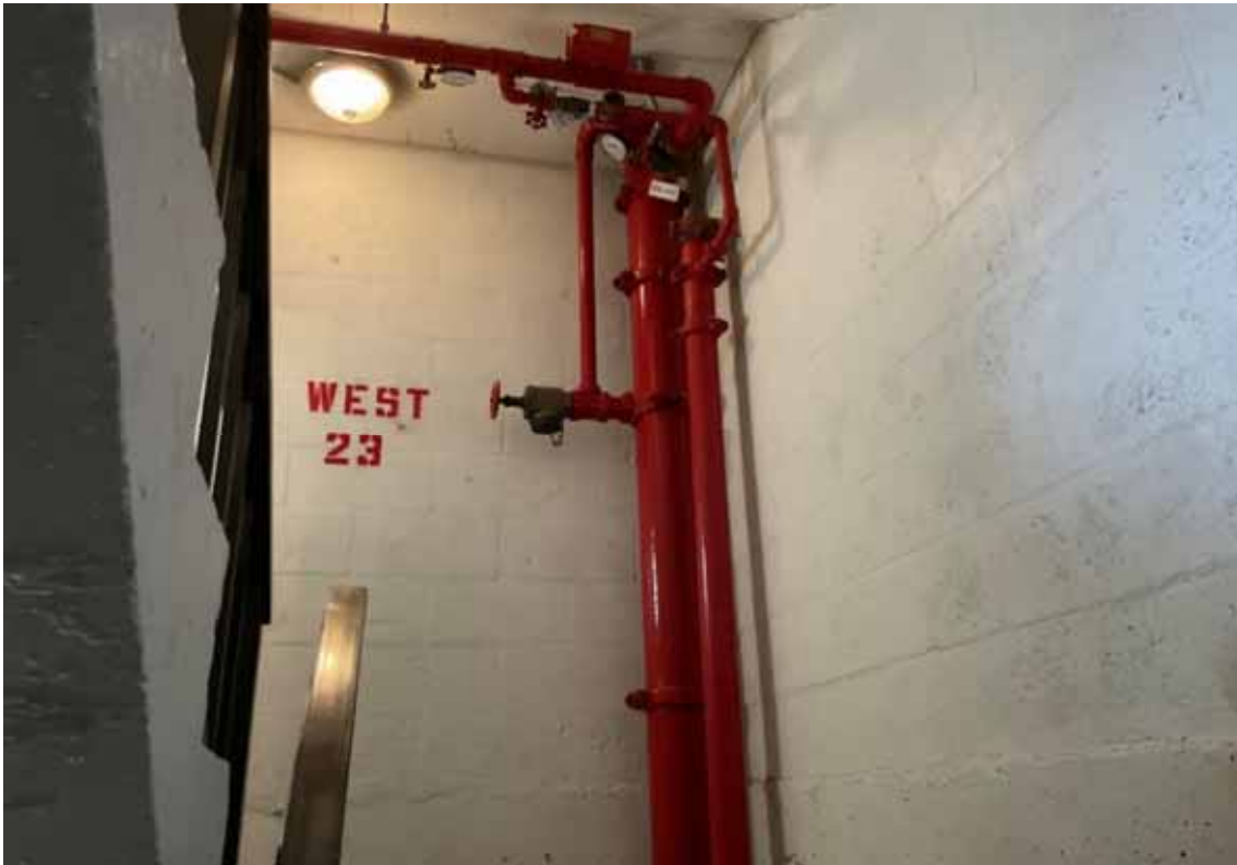
Bldg D Fire Standpipe
