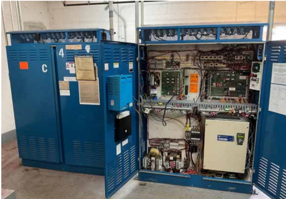
Bldg D Elevator Equipment
