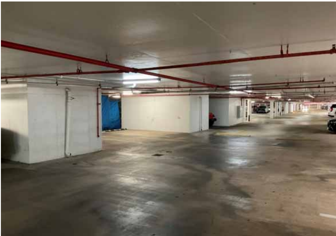
Garage Fire Sprinkler Lines
