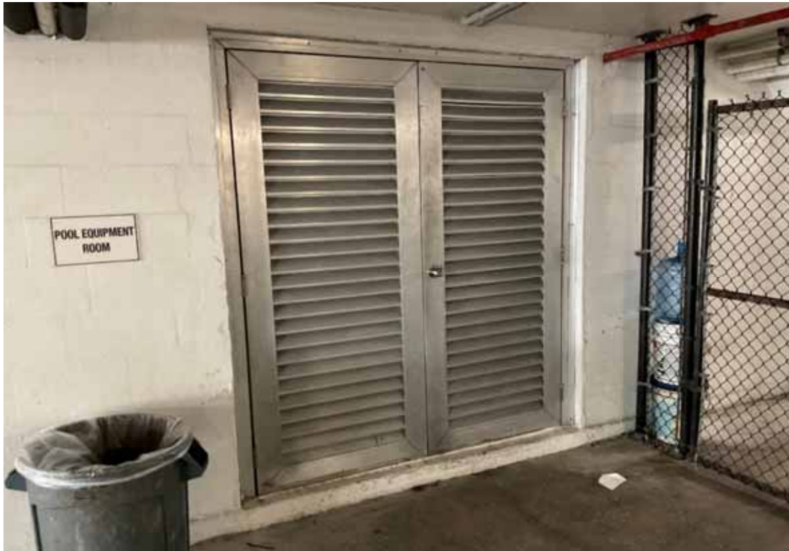
Doors - Pool Equipment Room
