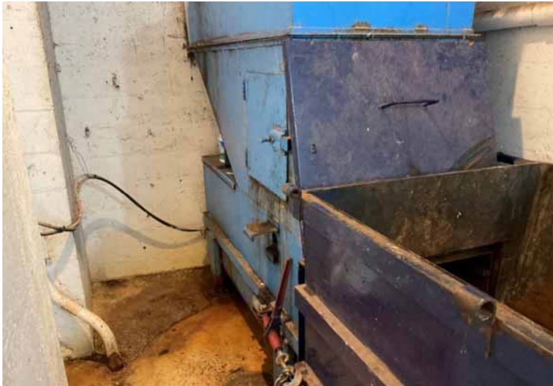
Bldg D Trash Compactor
