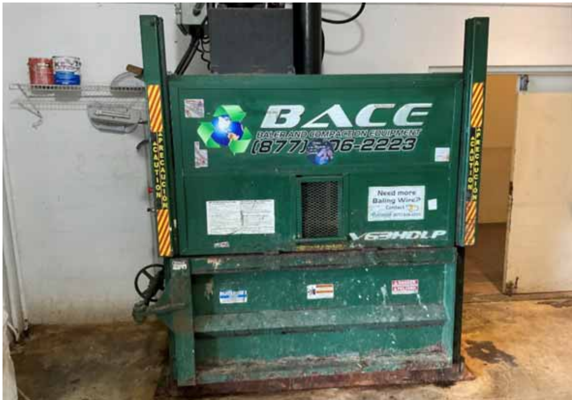
Bldg D Cardboard Bailer
