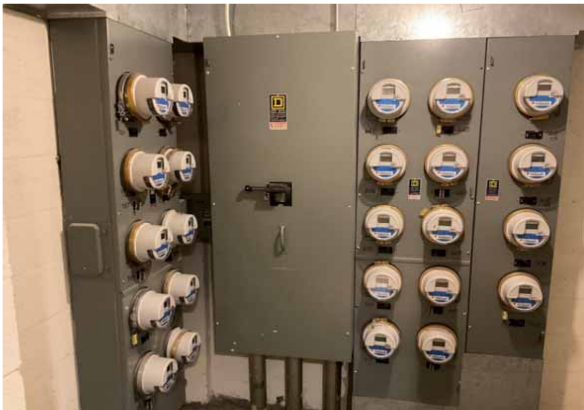
Bldg C Electrical Meters & Panel
