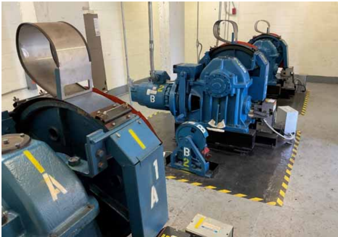
Bldg C Elevator Equipment
