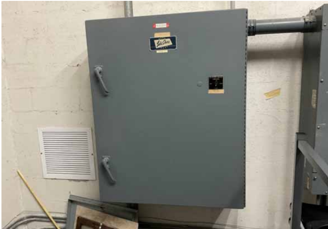
Bldg C Generator Automatic Transfer Switch
