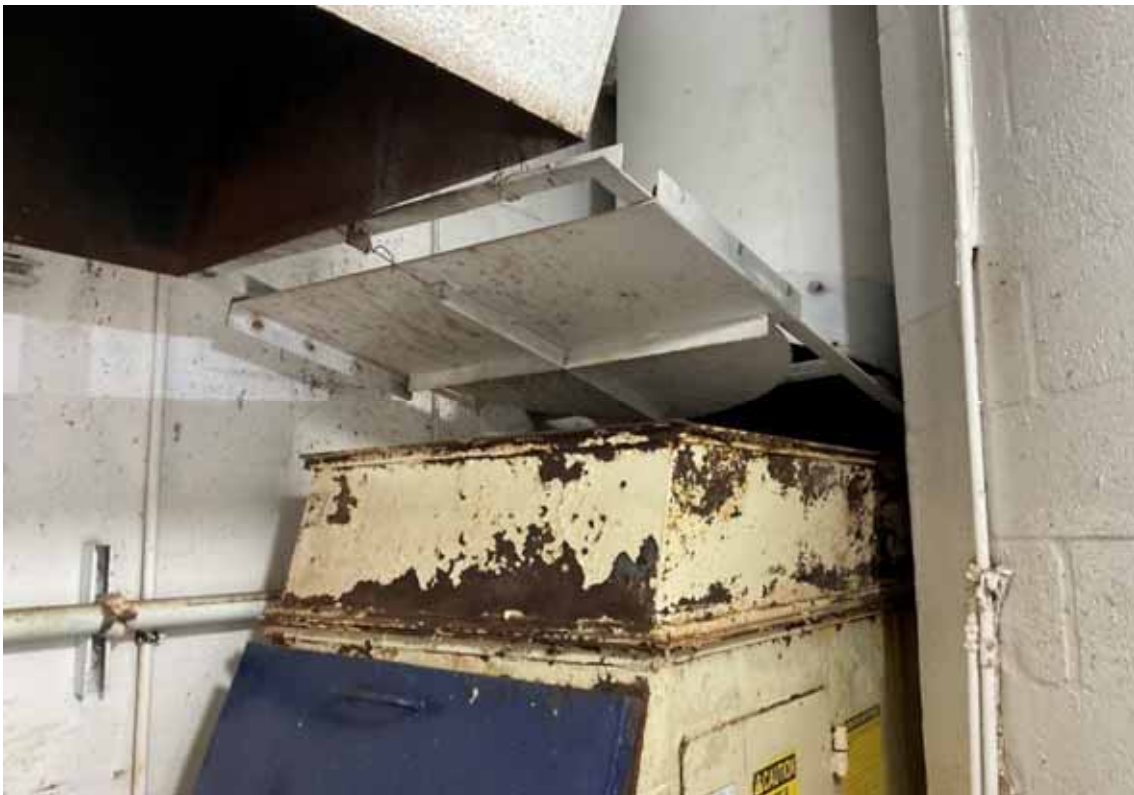
Bldg C Trash Chute Guillotine
