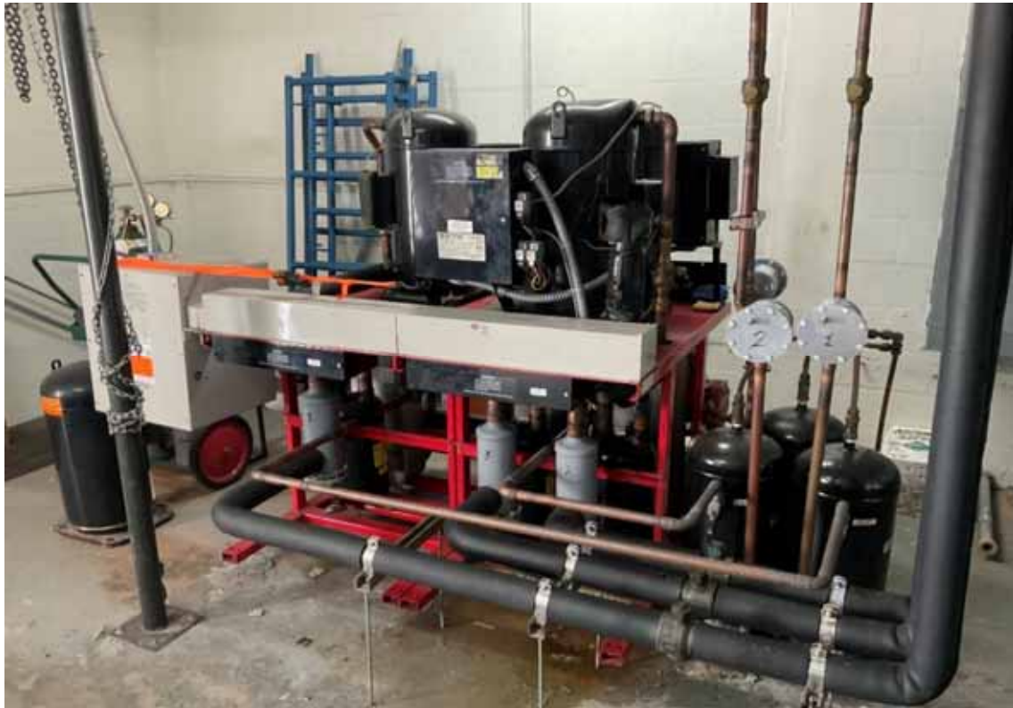
Bldg C A/C Compressor Unit
