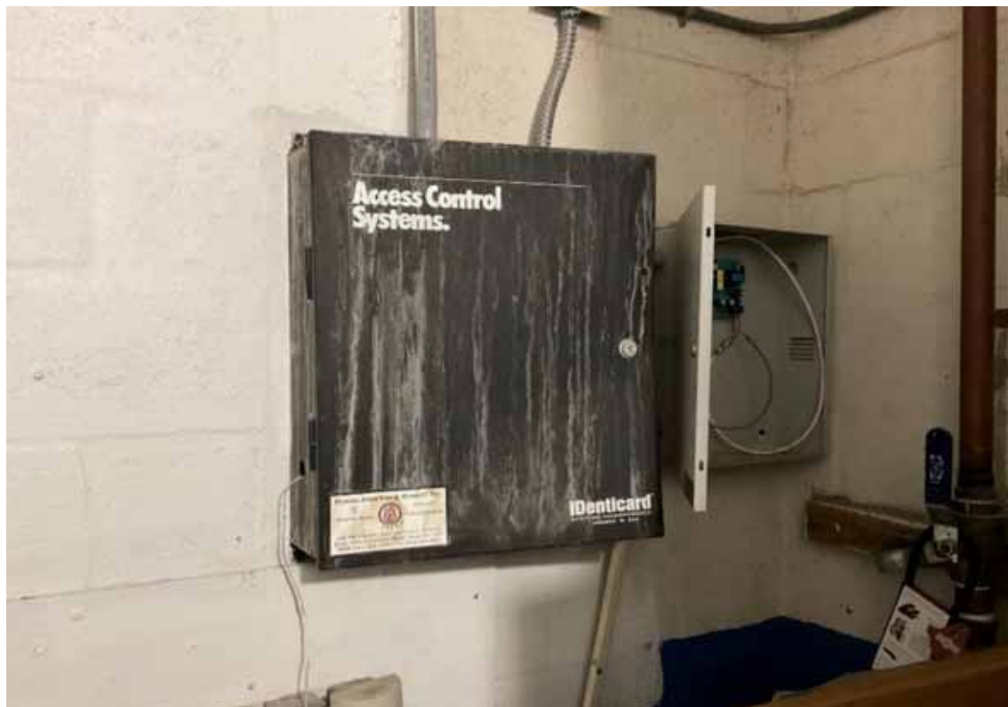
Bldg D Access Control Equipment
