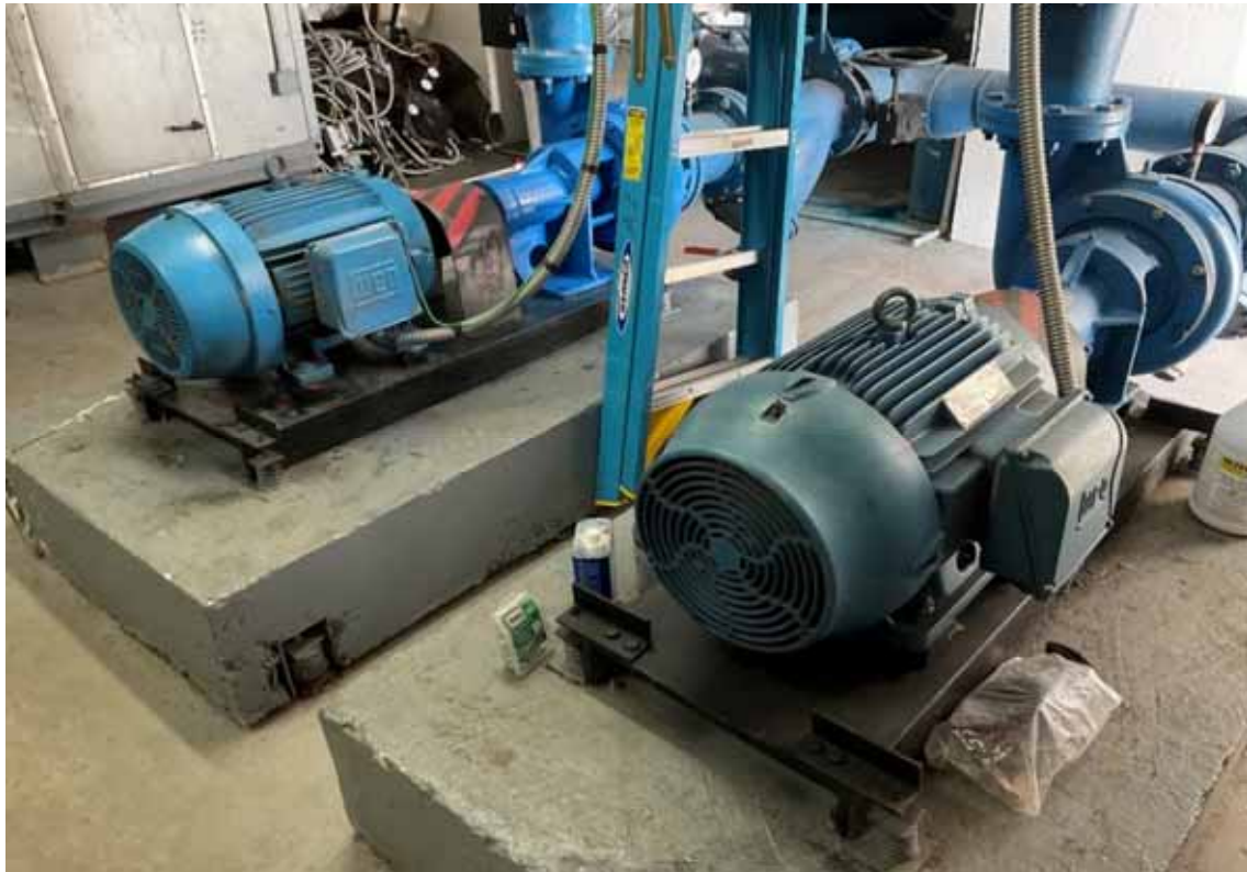
Bldg D A/C Condenser Pumps
