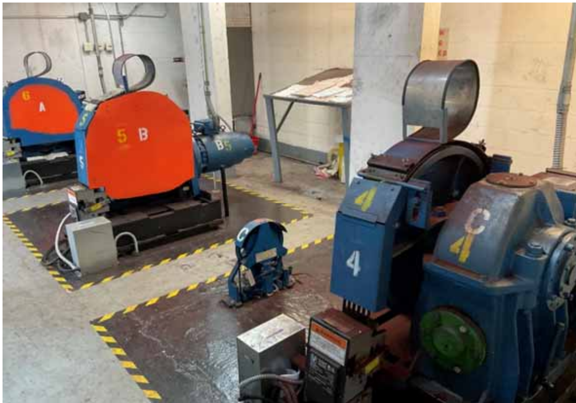
Bldg D Elevator Equipment
