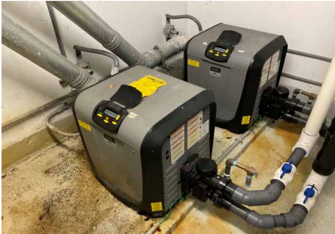
Pool Equipment, Heaters
