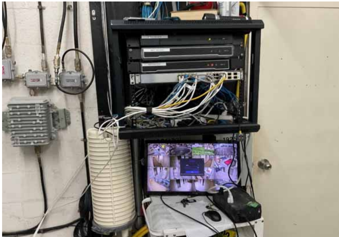
Bldg D Video Surveillance Equipment
