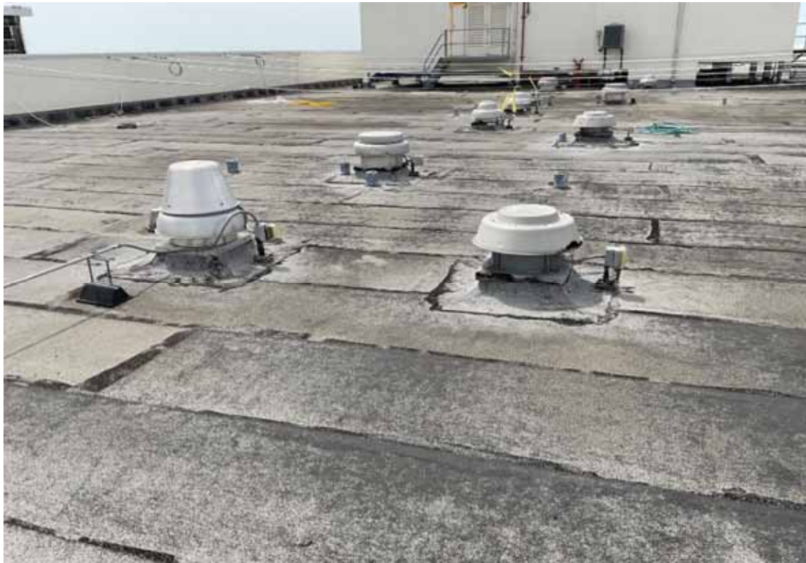
Bldg C Rooftop Exhaust Fans
