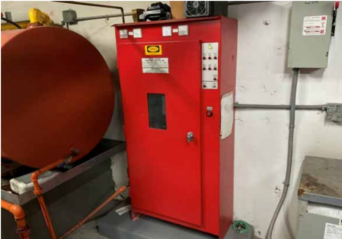
Fire Pump Controller
