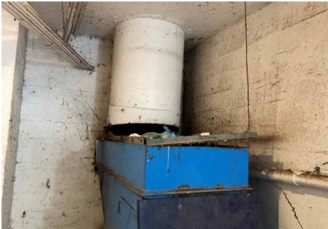
Bldg D Trash Chute Guillotine
