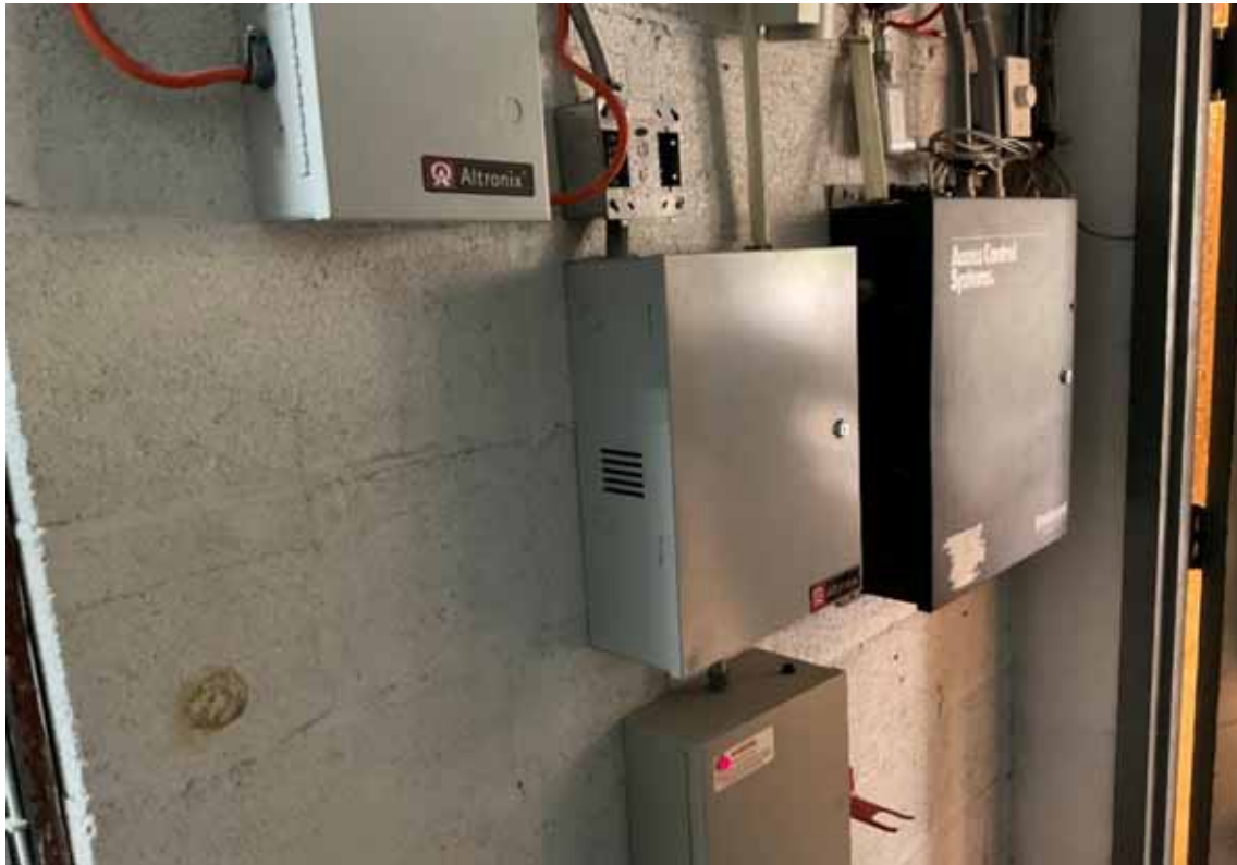
Bldg C Access Control Equipment
