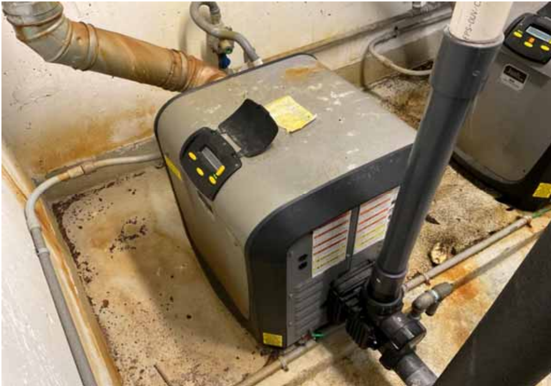
Spa Equipment, Heater
