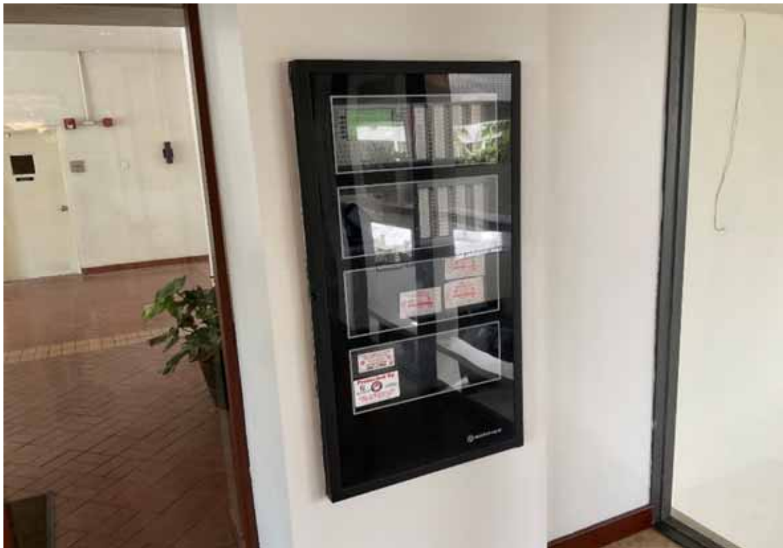
Bldg D Fire Alarm Panel
