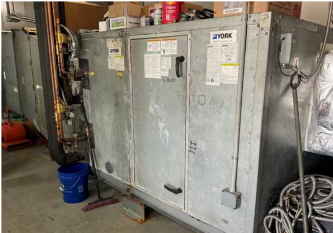
Bldg D A/C Air Handler
