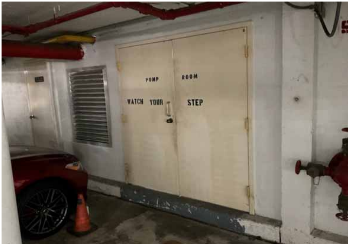
Doors - Pump Room
