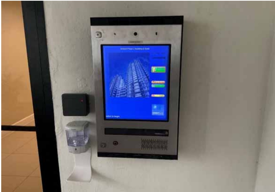
Bldg D Enterphone - 2nd Floor
