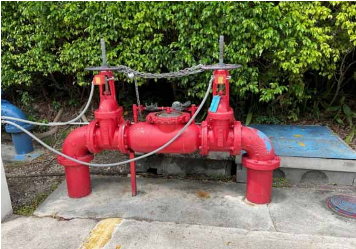
Backflow Preventer - Fire
