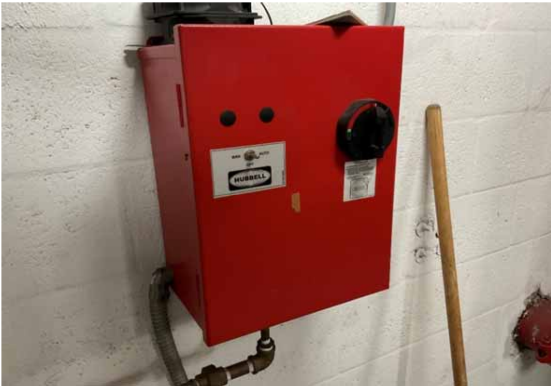
Fire Jockey Pump Controller
