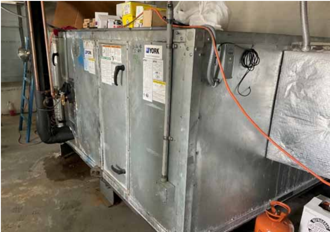
Bldg C A/C Air Handler
