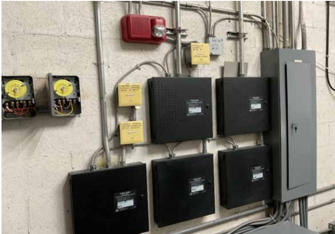
Bldg C Fire Alarm System Equipment
