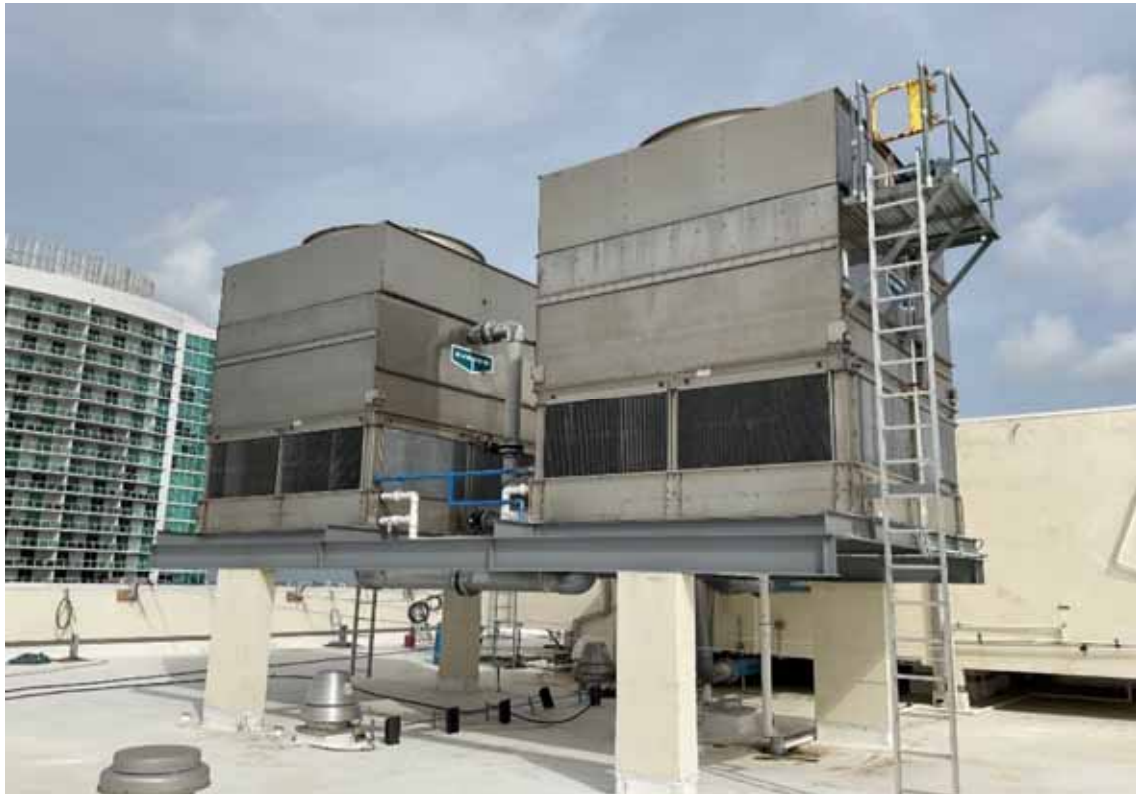
Bldg D A/C Cooling Towers
