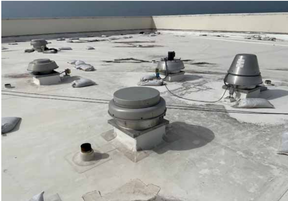
Bldg D Rooftop Exhaust Fans
