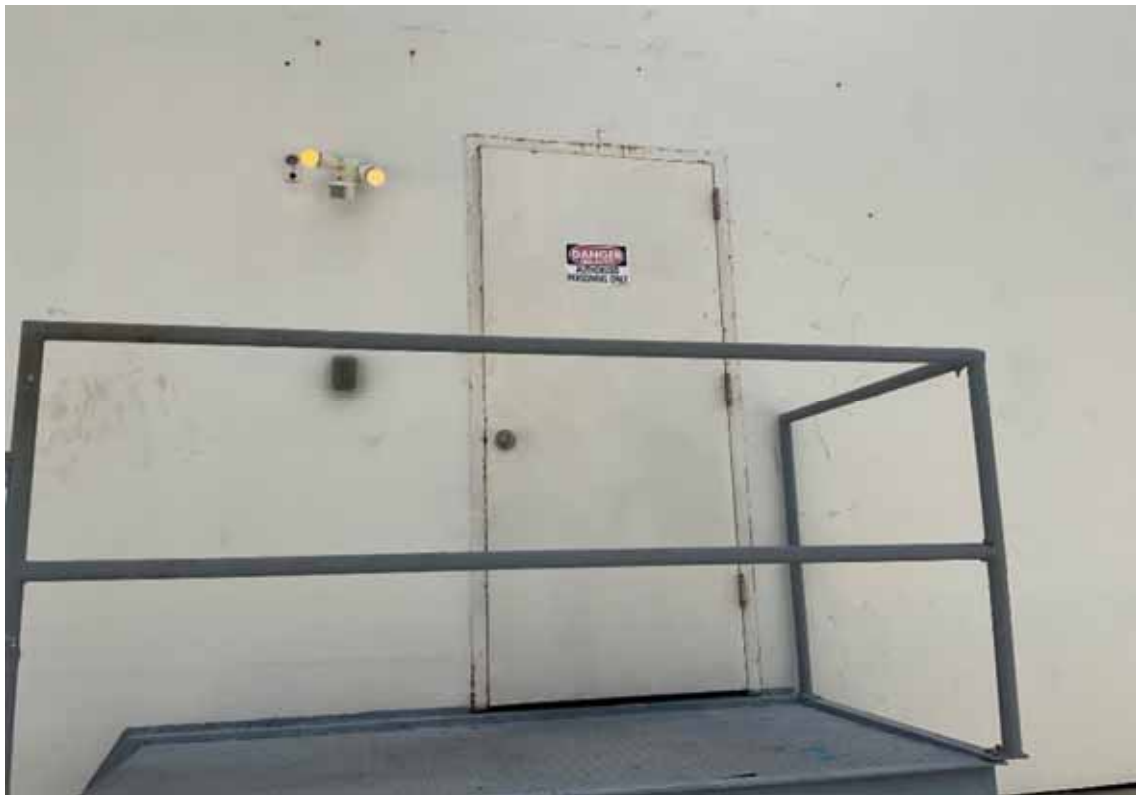
Door - Bldg D Elevator Equipment
