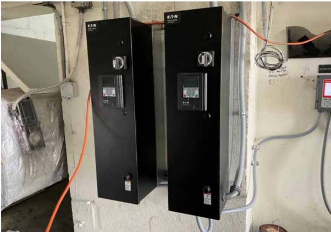
Bldg C A/C Cooling Tower VFD's
