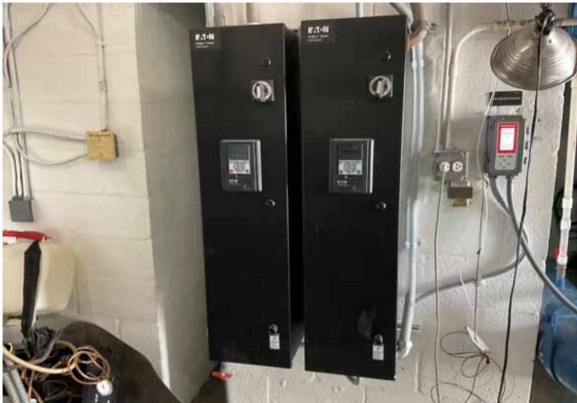
Bldg D A/C Cooling Tower VFD's
