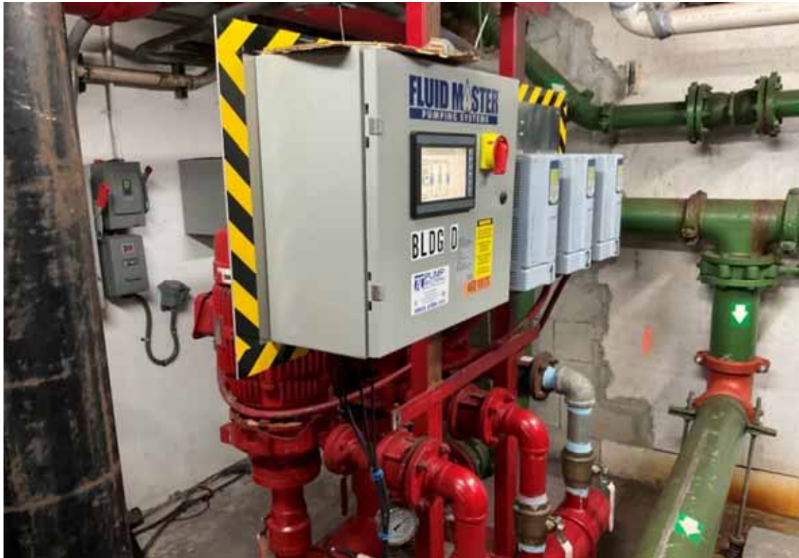
Bldg D Domestic Water Booster Pump System
