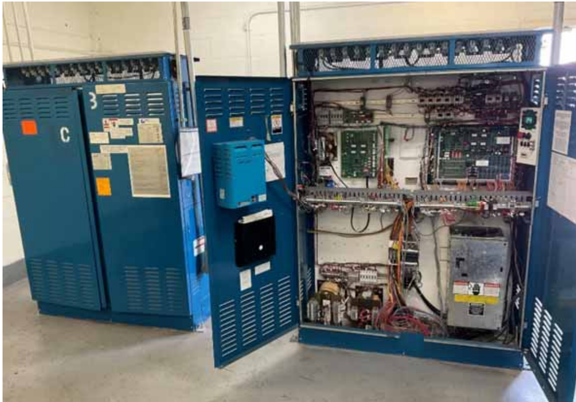
Bldg C Elevator Equipment
