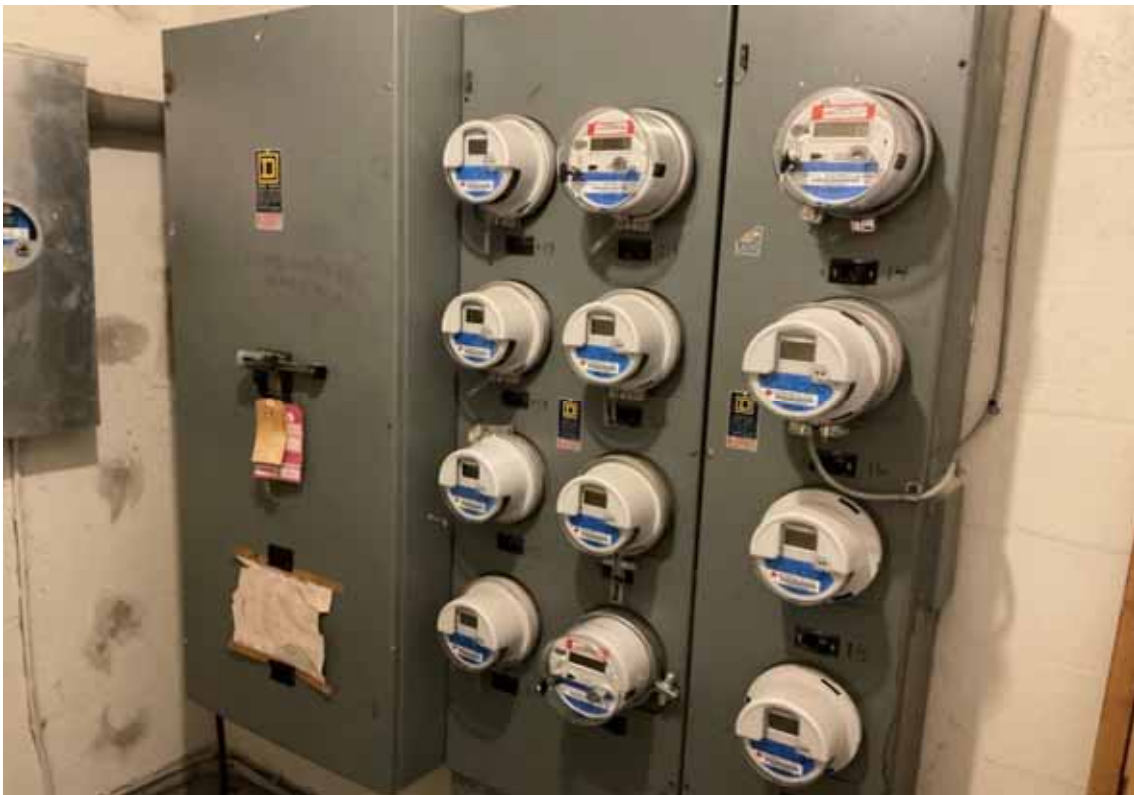
Townhouse Bldg Electrical Meters & Panel
