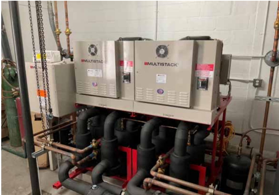
Bldg D A/C Compressor Unit
