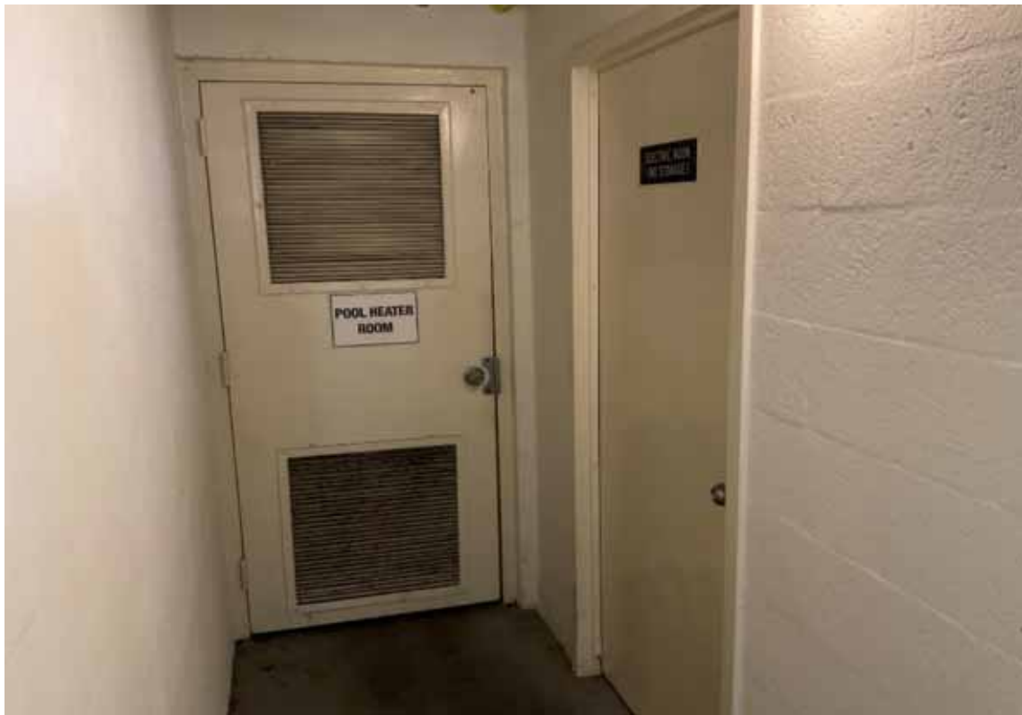
Doors - Pool Heater & Electrical Room
