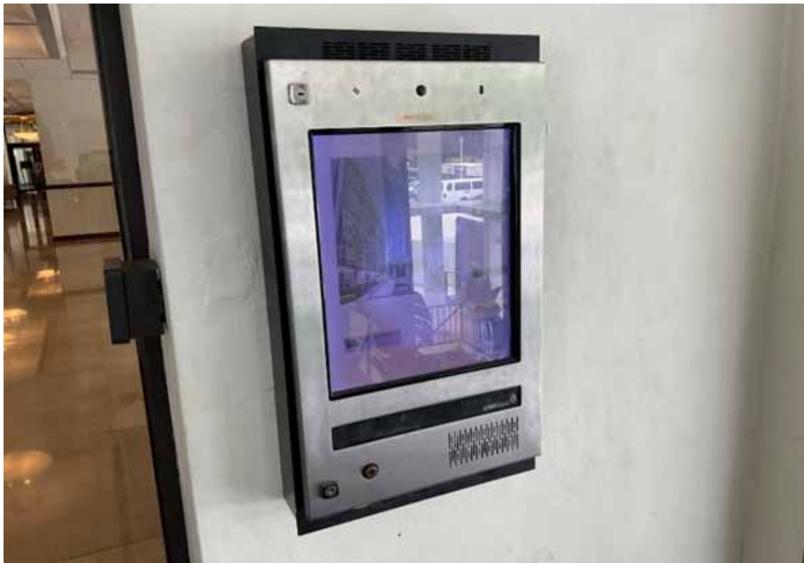
Bldg D Enterphone - Lobby
