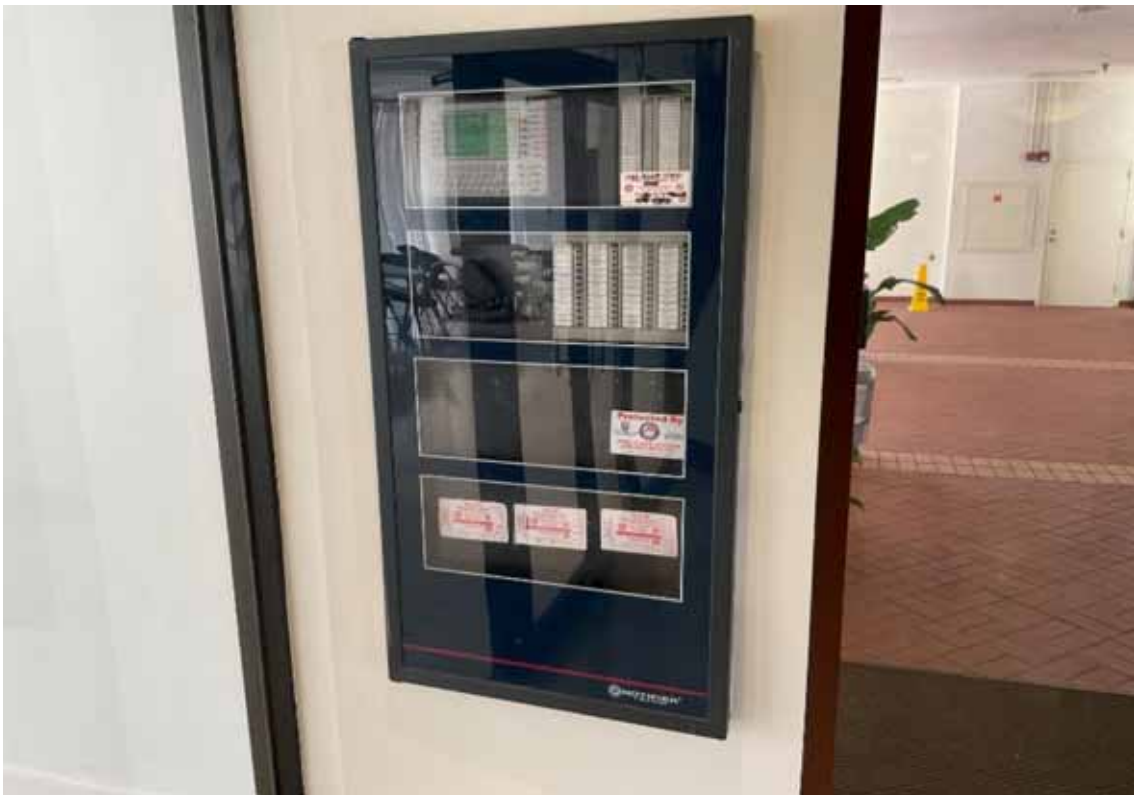
Bldg C Fire Alarm Panel
