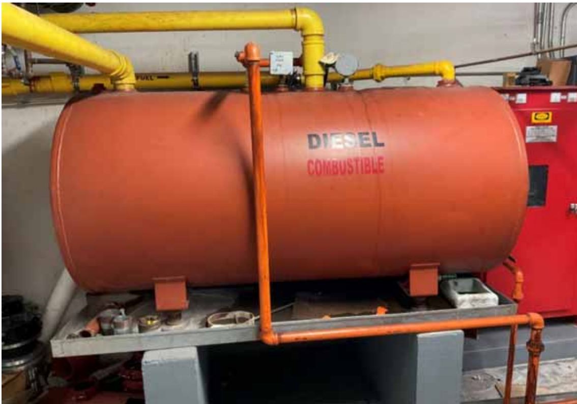
Fire Pump Fuel Tank
