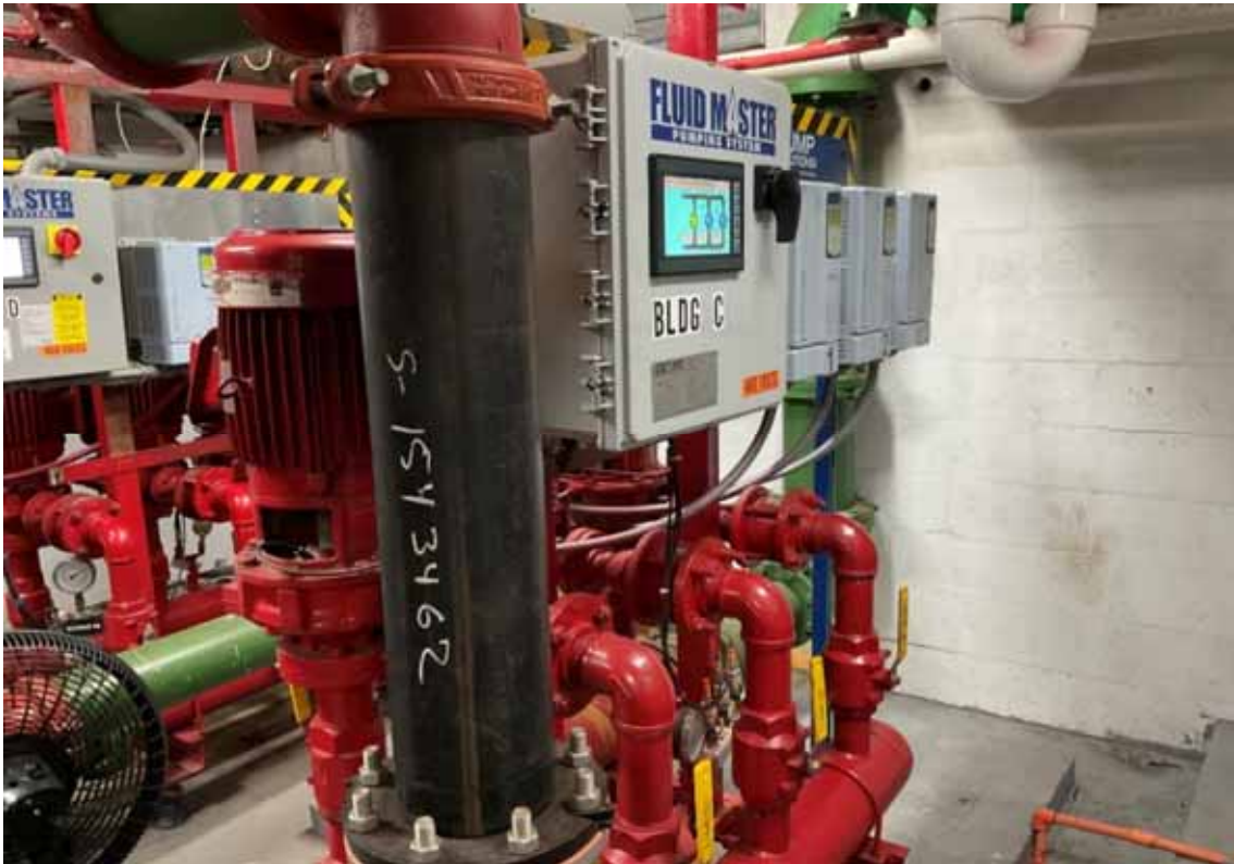
Bldg C Domestic Water Booster Pump System
