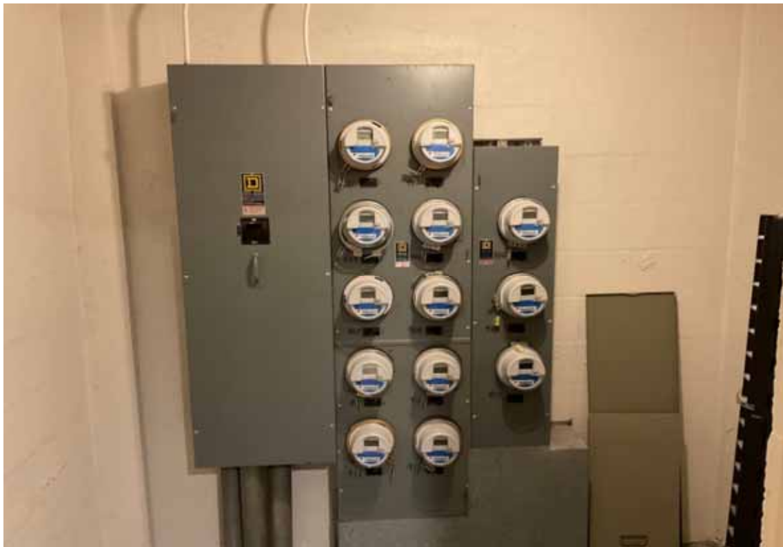
Bldg D Electrical Meters & Panel
