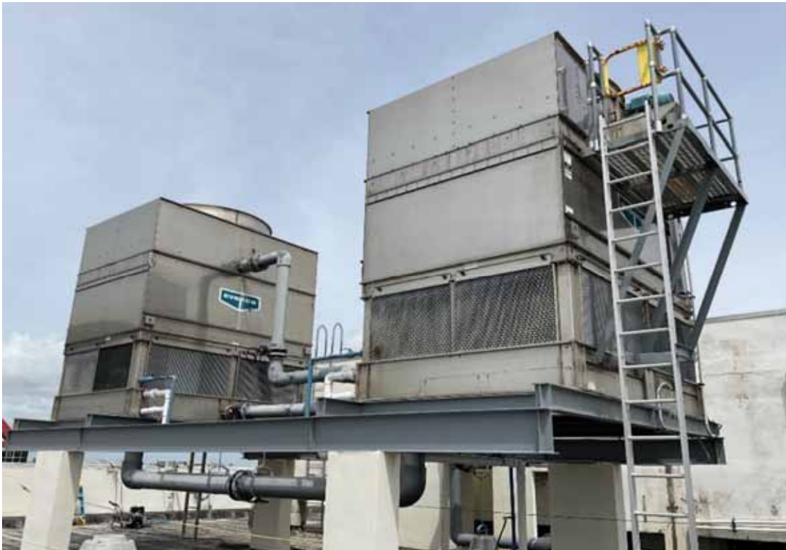
Bldg C A/C Cooling Towers
