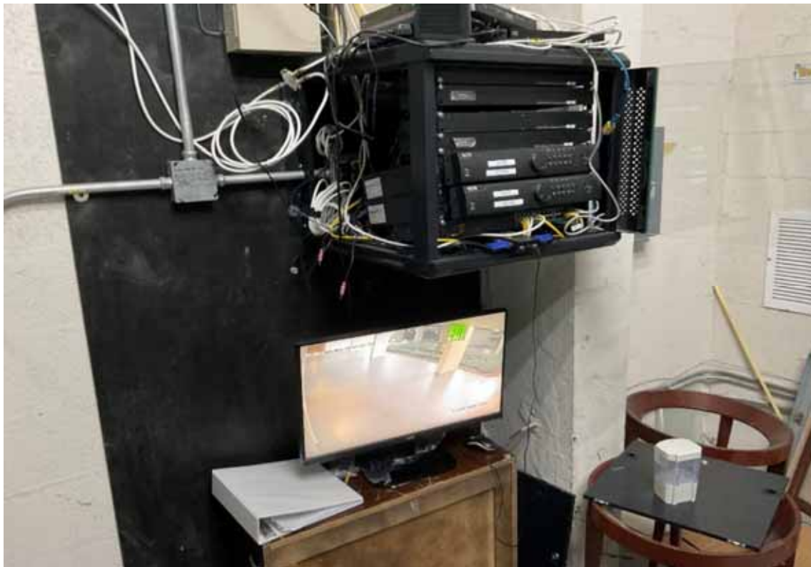
Bldg C Video Surveillance Equipment
