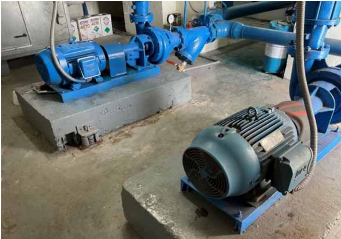
Bldg C A/C Condenser Pumps
